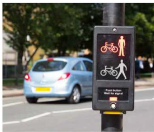
Nearside push-button control for toucan crossing
